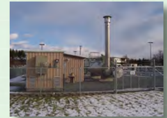
Metering and Regulating Station
