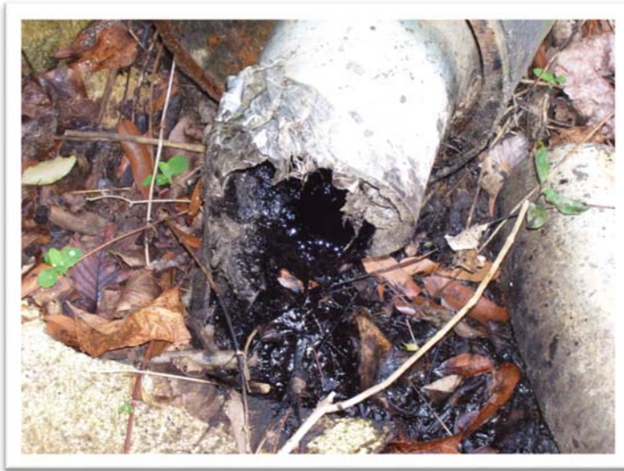
“Close-up” of oily substance discharging from pipe.
